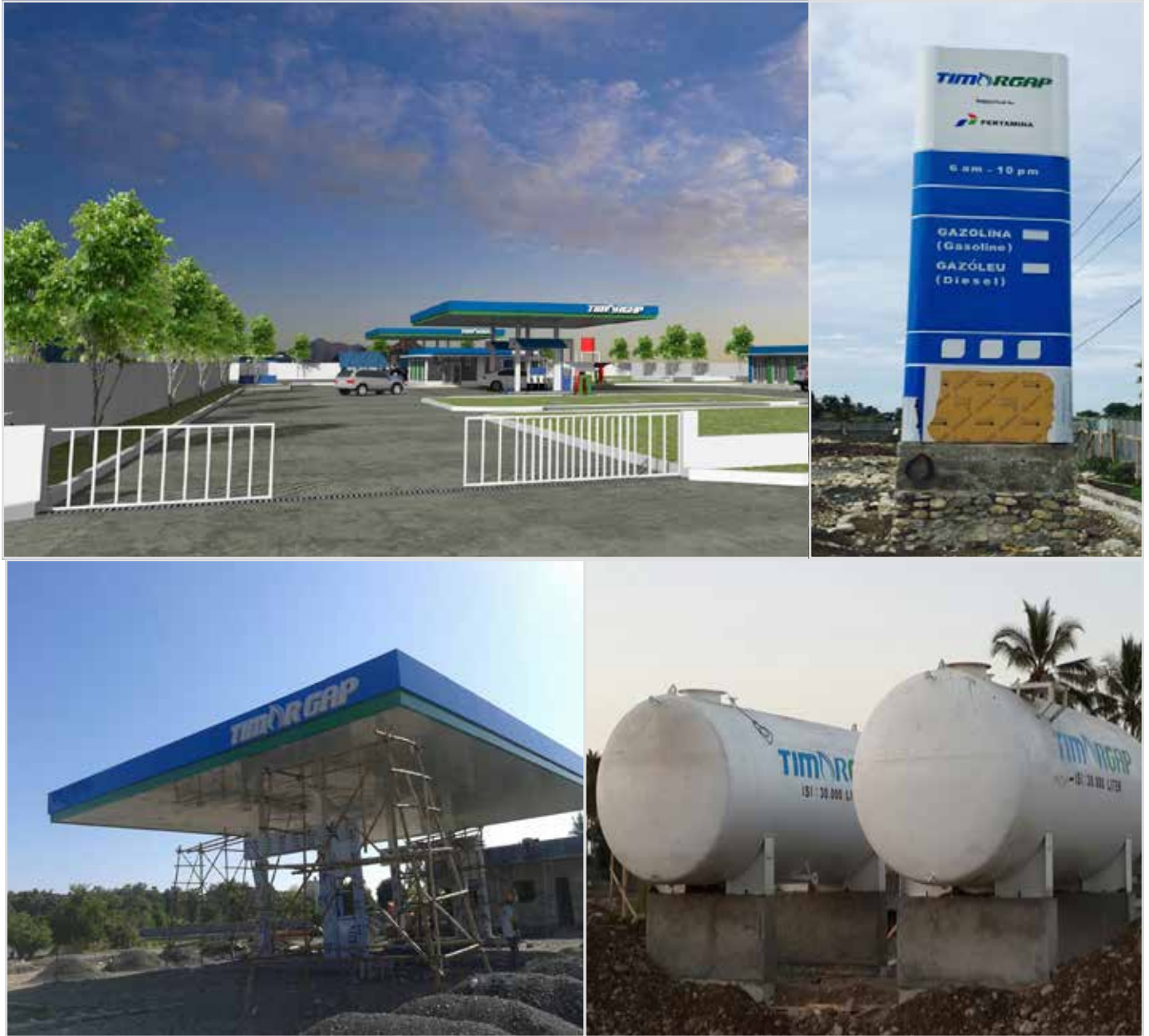
From top to bottom (left to right): Fuel station design; Fuel station and gasoil storage construction progress in Suai
