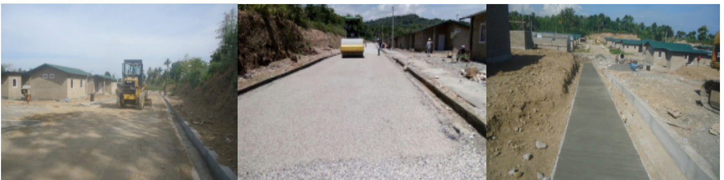
From top to bottom, left to right: New houses for affected community; Remaining houses under construction; Access road; Drainage system
