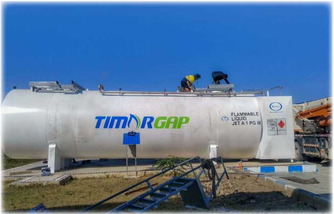
Figure 3-1: TIMOR GAP's fuel jet A-1 tank installation at Suai Airport
