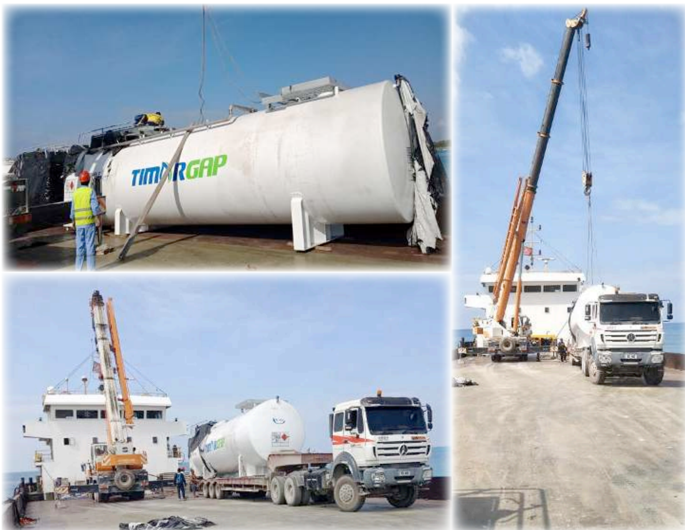
Figure 3-4: Jet A-1 fuel storage tanks unloading activities in the Suai port
