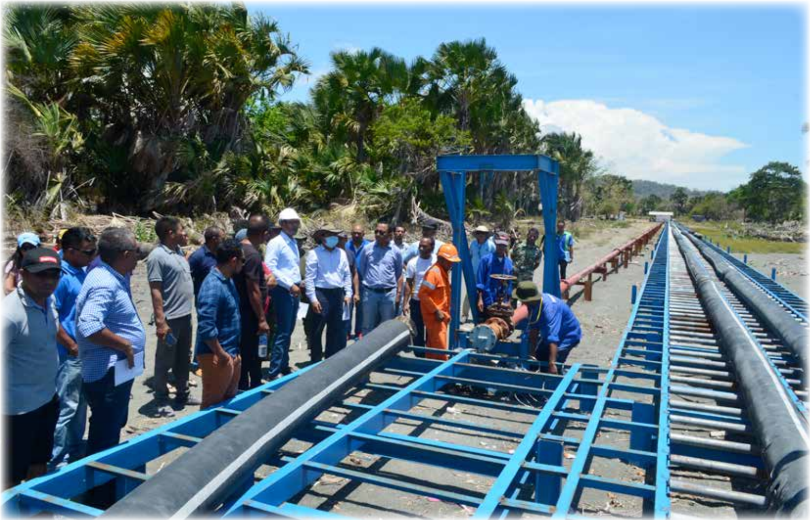
Figure 3-3: Visit of H.E. Minister of Petroleum and Minerals to SACOM fuel offloading facility in Betano
